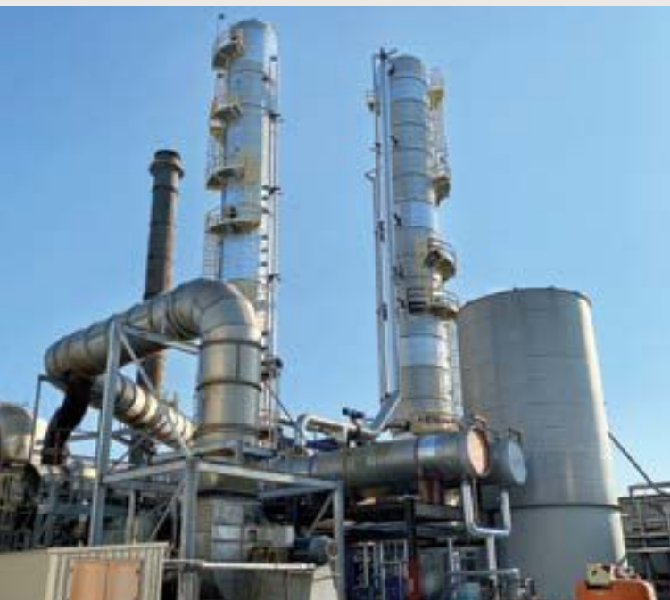
Below: York, Nebraska, ethanol plant with two distillation columns for a USP Grade alcohol system to make sanitizers and disinfectants.
