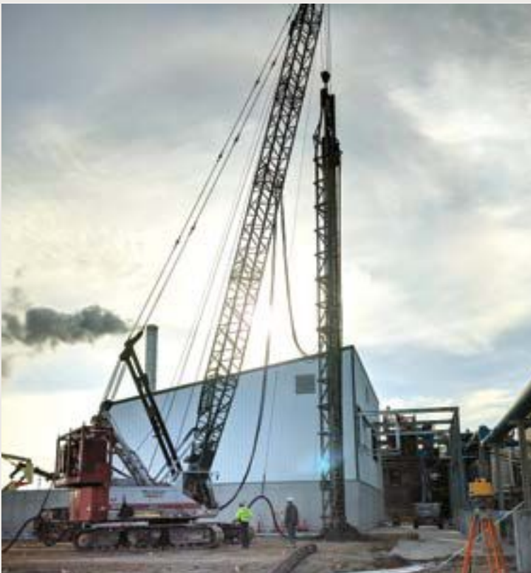
Above: Construction of FQT's MSC protein processing building, specifically the installation of a foundation pier, at an ethanol plant in Marcus, Iowa.
