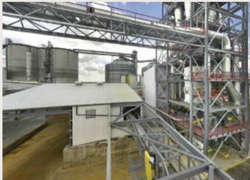
Below: The right side of the frame shows a ring dryer stack with wet pad in the foreground at a Marcus, Iowa, ethanol plant.
