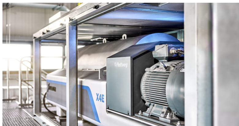
Two Xellektor X4Es are used for sludge dewatering at the main wastewater treatment plant.
