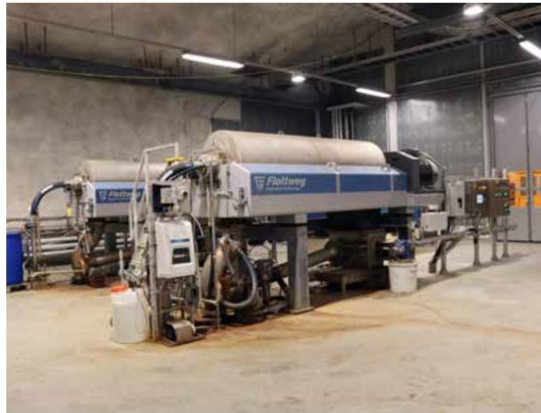
Two Flottweg C Series centrifuges handle the wastewater of the city of Turku.
