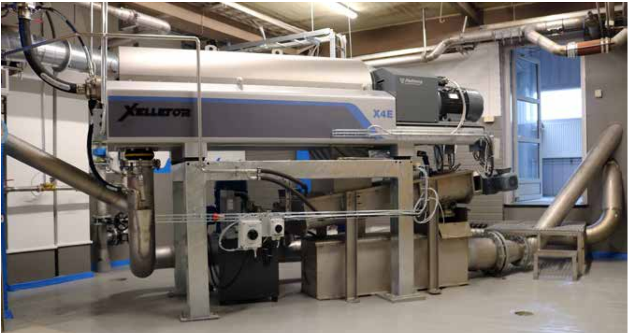
The Xellefor series in use in the Seinäjoki sewage treatment plant. The disposal costs were reduced by a quarter.
