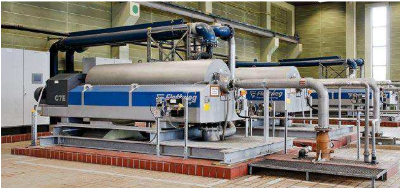
The decanter centrifuges at Flottweg in Vilsbiburg have been equipped with the Simatic S7-1200 fail-safe Basic Controller since the end of 2016
