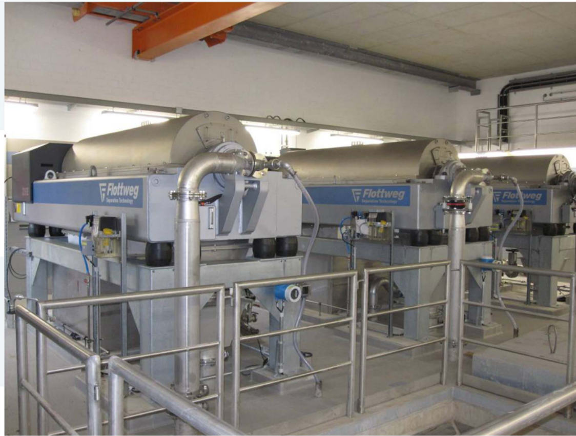
fig.: decanter plant
