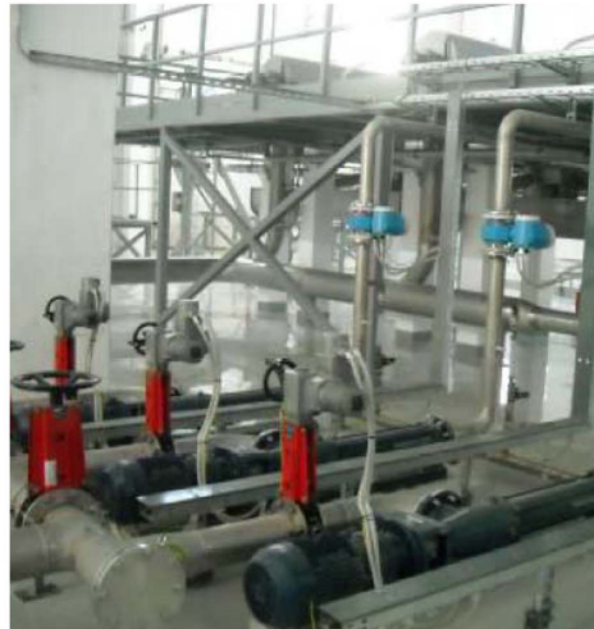
fig.: sludge pump unit
