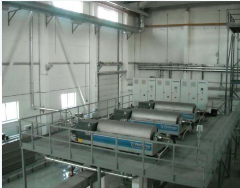
fig.: decanter plant
